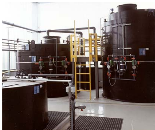
Neutralization and storage tanks for chemicals
